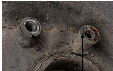
Cracks at Spring Plate Mounts
